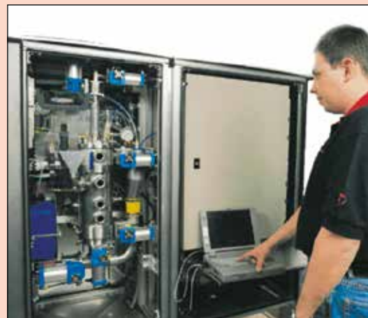
Valves and actuators for analyzer.
